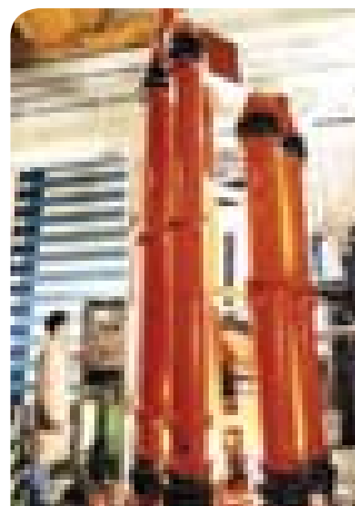
ICRF transmission lines at the ASDEX Upgrade tokamak
